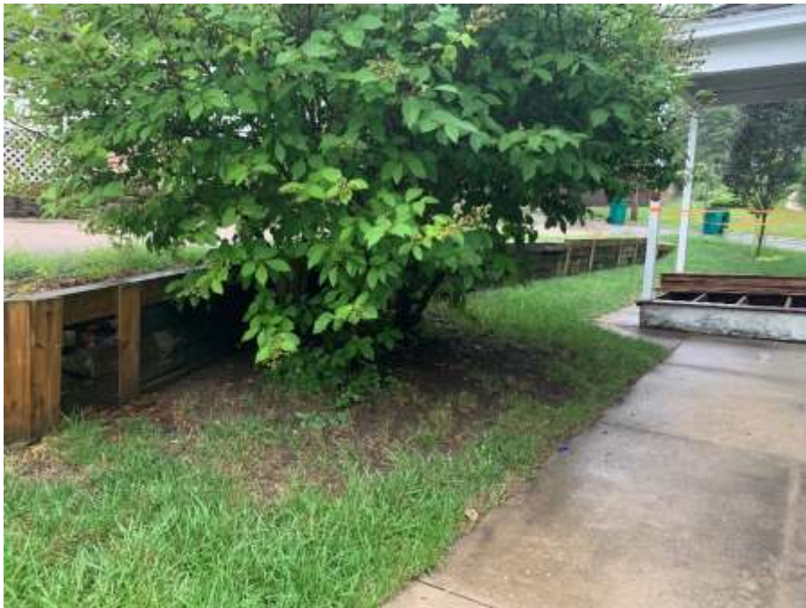
Image 2: Photo taken facing southwest. Lighter wood areas represent temporary stabilization measures added in past couple years to extend the life of the wall. Timbers closest to Third St are completely rotted and the area is not supported.
